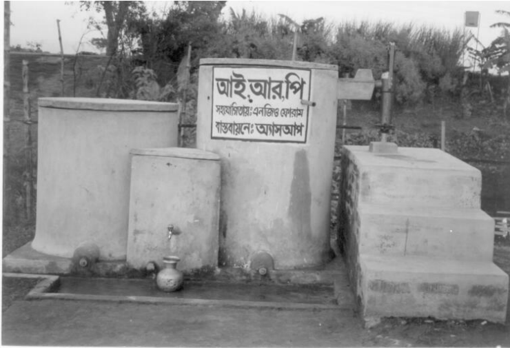
Figure 3. Small Community Type Arsenic and Iron Removal Plant
